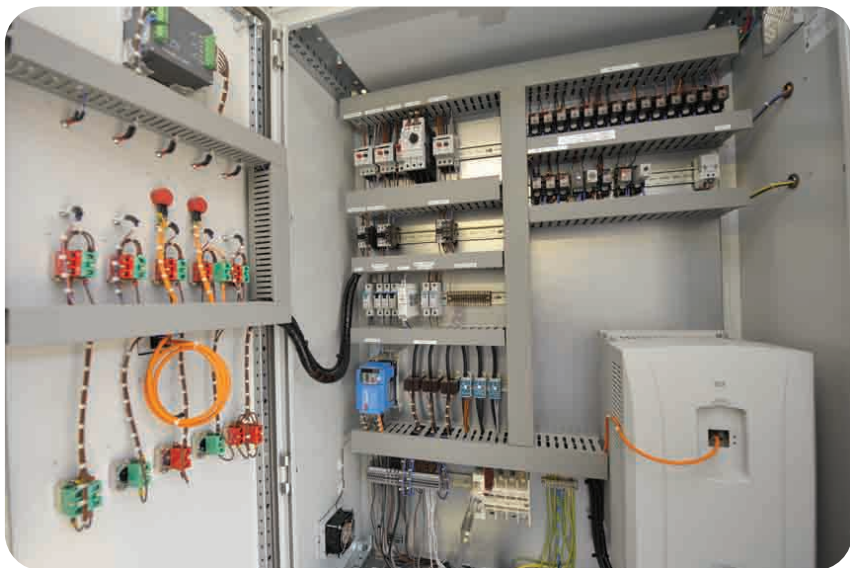
↑ Inside control panel with speed control inverters.
